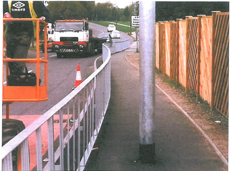
A new lighting column and pedestrian barrier combine to make the footway impassible
